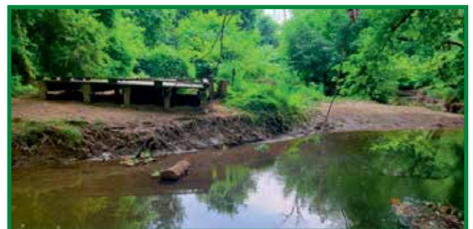
An eroded bank and prospective site for Stream Stabilization (downstream from the Paxton Creek Bridge)
